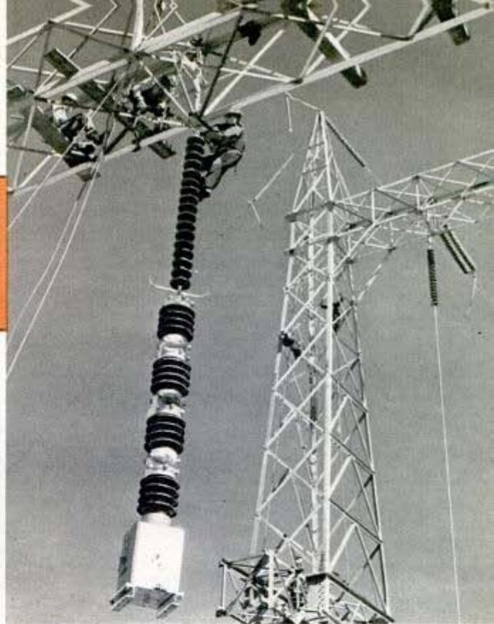
Here workmen are erecting an electric switching station. Every part of the power line from the dam to Vancouver, Seattle and Tacoma must be fully protected by automatic relays
